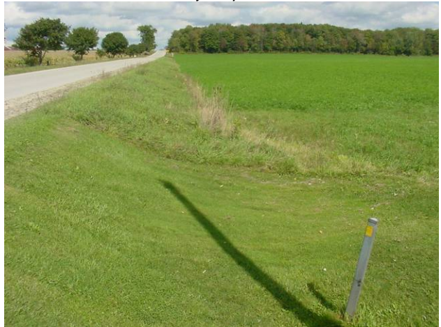
Plate 64: view to northeast, fill slope disturbance along the southeast side of McNabb.
