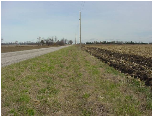
Plate 27: view to northeast, fill slope disturbance along Manley Line.
