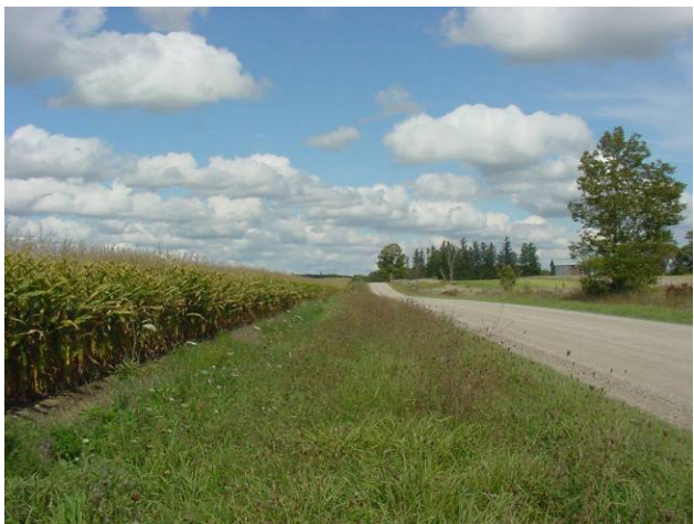
Plate 81: view to northeast, ditch and fill slope disturbance along McNabb Line.
