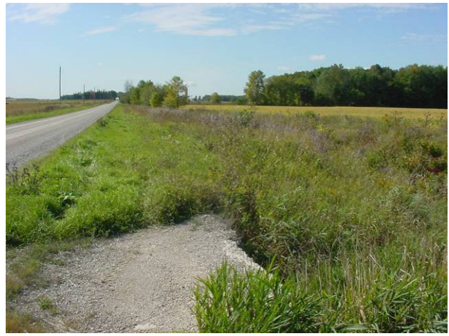
Plate 28: view to southwest, fill slope disturbance and deep drainage ditch along Manley Line.
