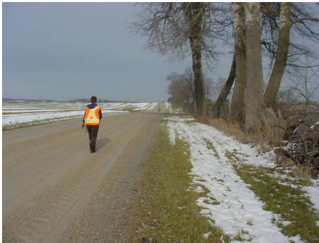
Plate 67: view to northeast, fill slope disturbance along McNabb.
