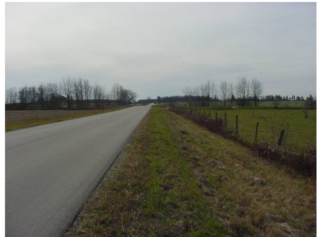
Plate 44: view to southwest, fill slope disturbance along paved and improved McNabb. Low and level terrain near channelized stream.
